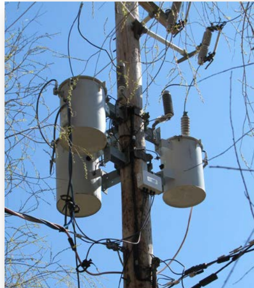
Figure 2: LineWatch-L sensor integrated with a three-phase pole-mounted distribution transformer installation.
